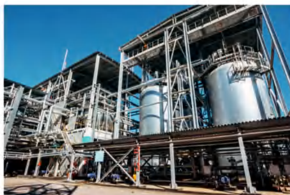
A structure of application - Reaction Tank
