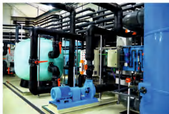
A structure of application - Desalination Plant
