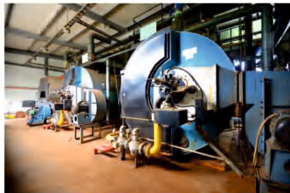
A structure of application - Boiler
