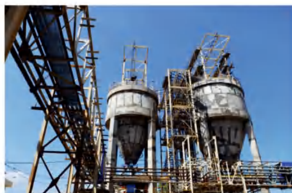
A structure of application - Ash Handling Plant
