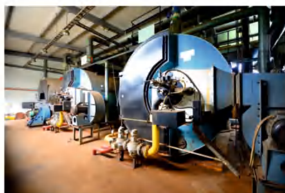
A structure of application - Boiler
