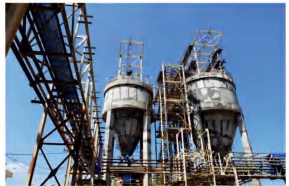
A structure of application - Ash Handling Plant
