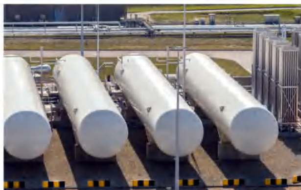
A structure of application - Gas Storage
