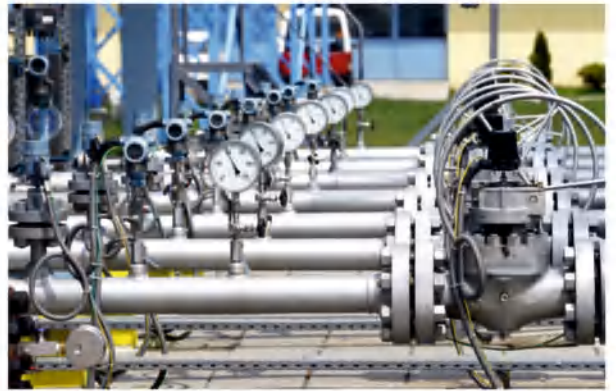
A structure of application - Fuel Gas Transmission
