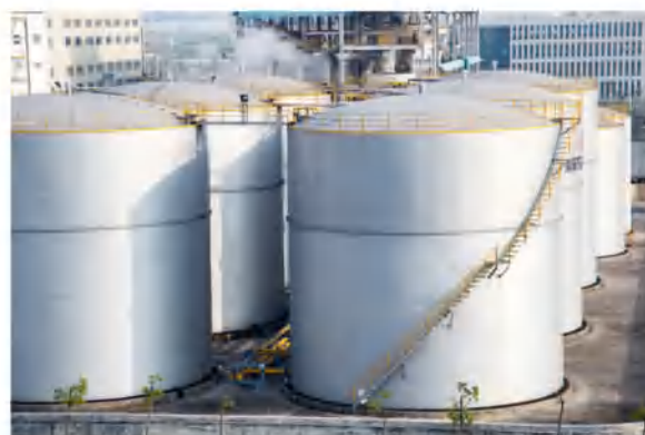
A structure of application - Reaction Tank
