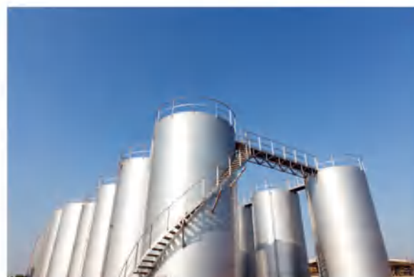
A structure of application - Reaction Tank
