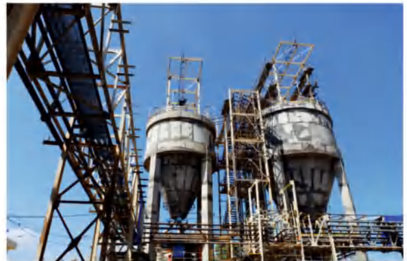
A structure of application - Ash Handling Plant
