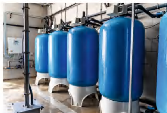
A structure of application - Desalination Plant
