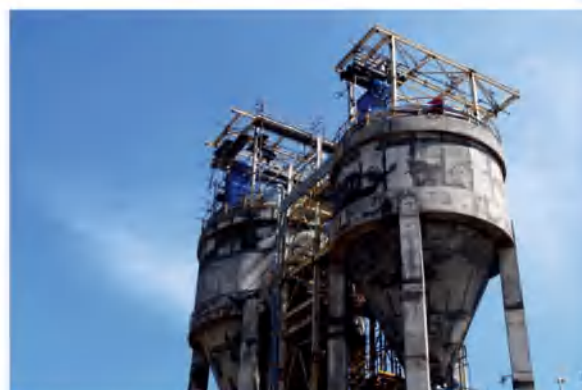
A structure of application - Ash Handling Plant
