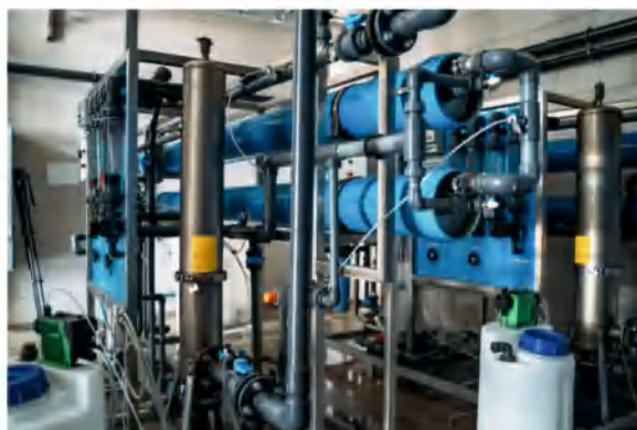
A structure of application - Desalination Plant
